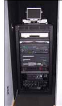
Far left: The 4 th floor conference room rack is recessed into the customer's cabinetry.
