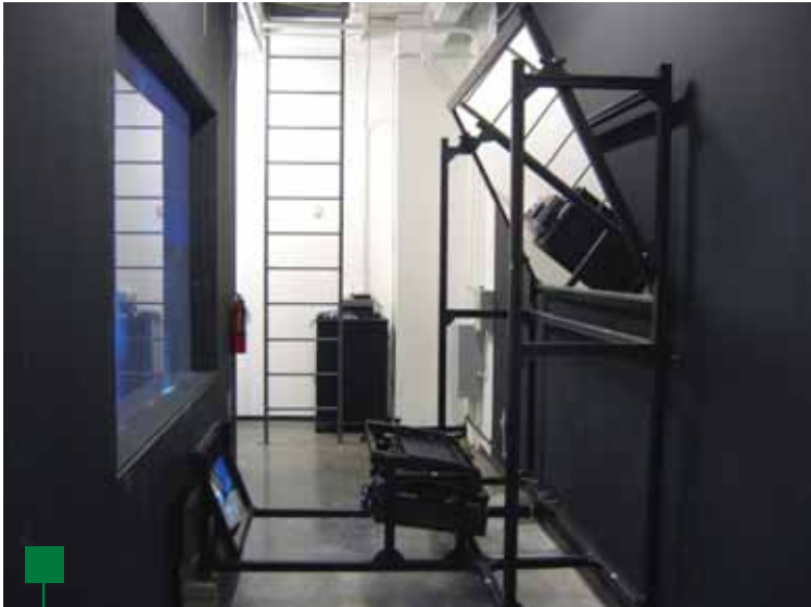
This custom rear projection module allows for the museum's 133-inch screen to be filled while requiring only nine feet of space. These modules were also used in both of the large conference rooms.
