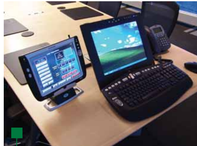
Total system control is provided at the head of the conference table. For convenience, the wireless touchpanel can be removed from the cradle for system operation anywhere in the room. The ability to operate PC applications and annotate over content is available through a wireless keyboard, mouse and interactive pen display. An IP telephone set is available for company voice communications.
